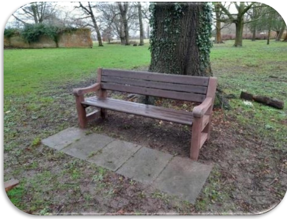
Figure 21: NE87– To fund the removal of the dilapidated bench beneath and replace with a 4 seat maintenance-free bench on Woodmansterne Village Green.
