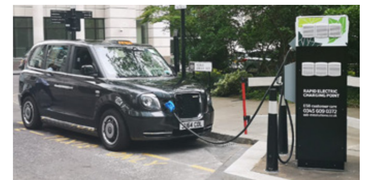
Image 4.7: Example of EV charging point
